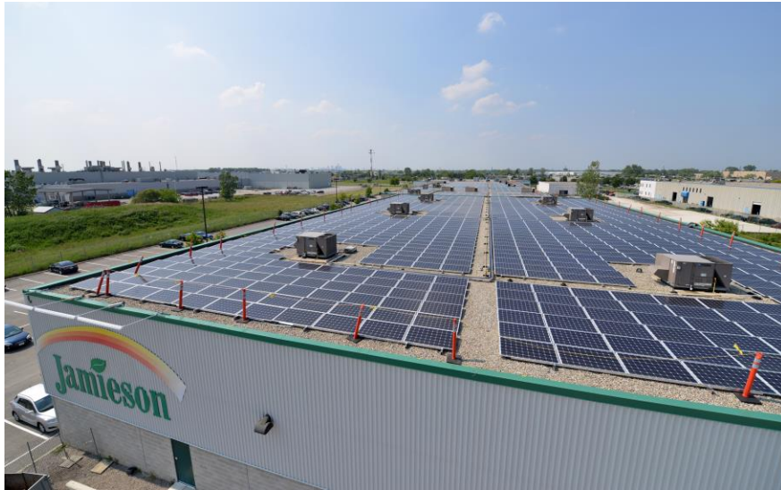
Solar panels on the roof of Jamieson's manufacturing facility in Windsor, Ontario
